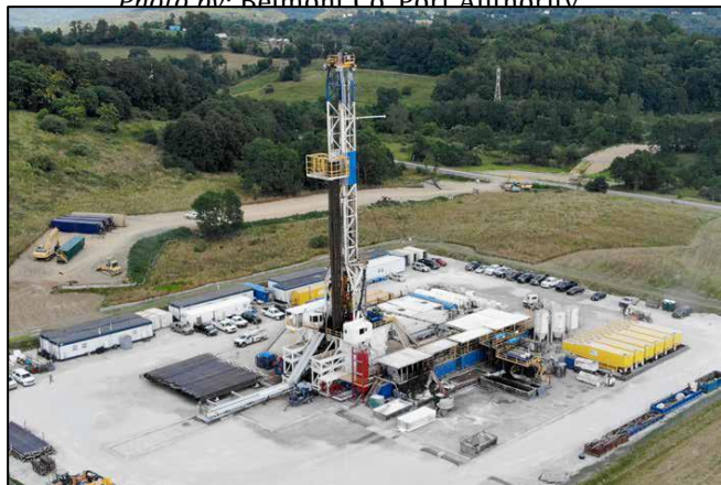
An Appalachian Marcellus/Utica shale Drilling Rig and pad. Photo by Ohio Oil & Gas Association
