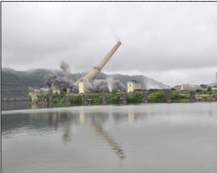
The R.E. Burger plant smokestack demolition in 2016. Photo by Times Leader's Joe Lovell
