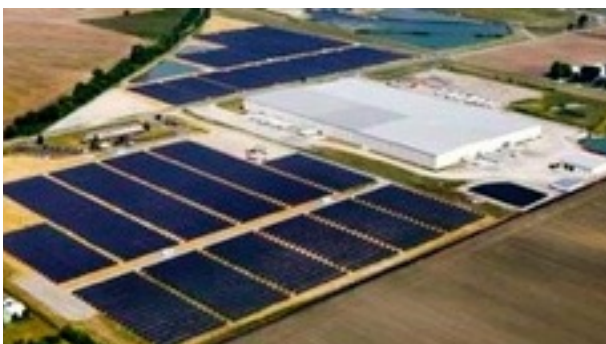
Campbell Soup Co. installed a 9.8 Megawatt Solar field designed to offset more than 15% of their electric consumption at their Napoleon Facility.
